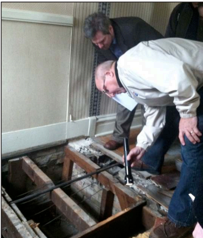
Doug Kline of American Home Improvements, Inc., and Executive Director Bill Firstenberger examine the revealed service stairway leading to the Robert and Peggy Weed Dining Room Gallery.
